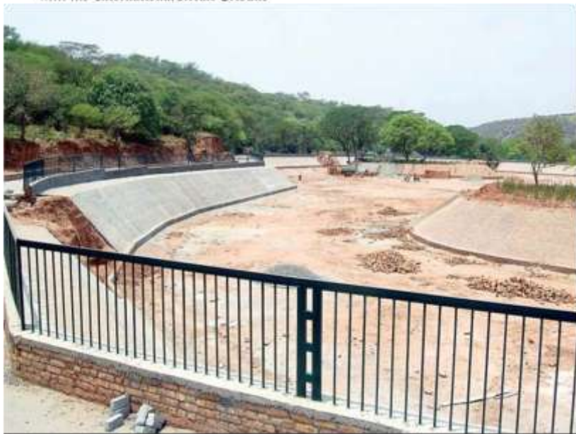
A view of an artificial lake under construction (left), broken animal statues in the children's play area (right) at the Lohi Bher Wildlife Park. PHOTOS: MUHAMMAD JAVAID
